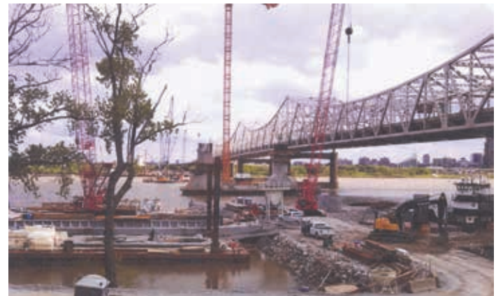
Walsh Construction working on Section 2 of the Downtown Ohio River Bridge on the Indiana side
