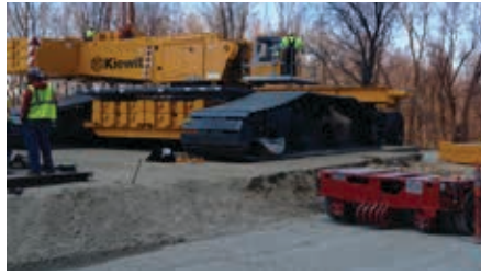
Above and Right: Assembly of the LR1750 Liebherr Crawler Crane that Kiewit is using on their environmental controls project at IP&L Power Plant in Petersburg, Indiana
