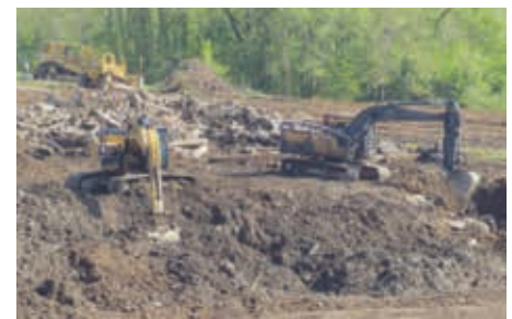
Phillips and Jordan site work at TVA for the Natural Gas Combined-Cycle Generating Station
