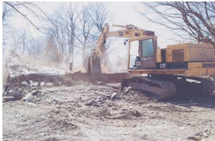
Now that old buildings are down and the clean-up is over, the Gibson County Habitat for Humanity can start the launch of five Habitat homes this fall. Thanks to all the hard work our journeymen and apprentices put in.
