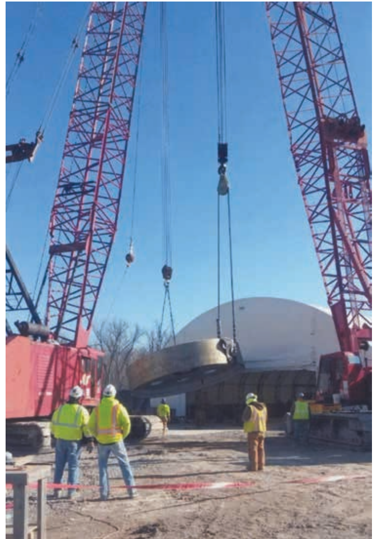
Operators Brad McGullion and Dave Newton for C.J. Mahan at the Smithland Hydroelectric plant rotating turbine parts
