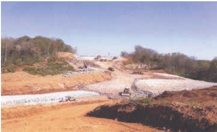
Bloomdsale Excavating on the I-265 grade and drain extension to the East End Bridge
