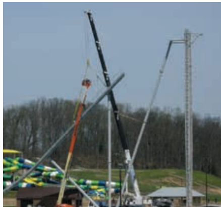
General Steel taking down a ride at Holiday World for Deig Bros.
